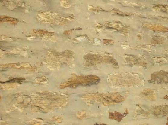
Poor cement pointing that over dominates the stonework and can hasten the deterioration of the stone
