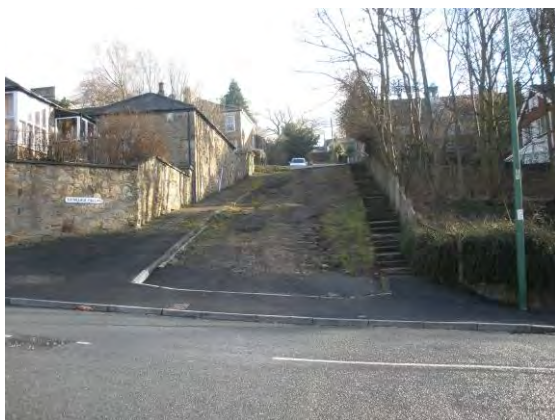
Kiln Bank - poorly surfaced leading to the Village Hall
