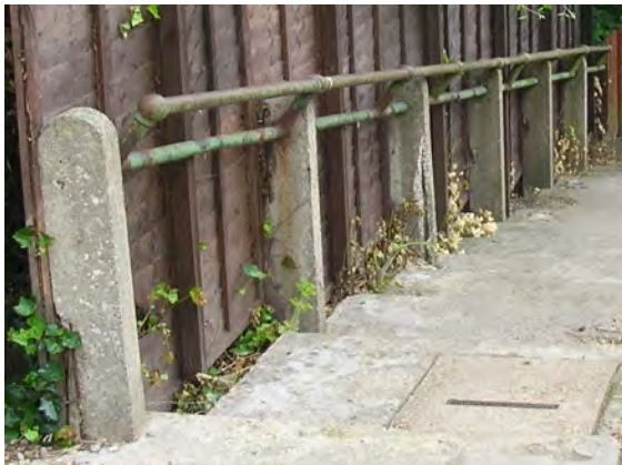
Standard modern railings that do not consider the character of the conservation area.
