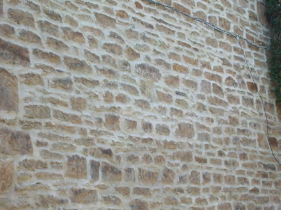
Good quality lime mortar pointing that respects the stone and allows it to breath
