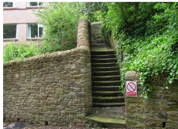
Steps on Church Bank – in need of repair and restoration
