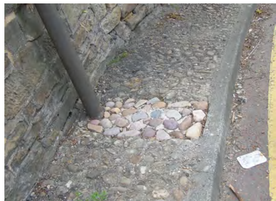
Example of where highway repairs have been carried out using inappropriate materials
